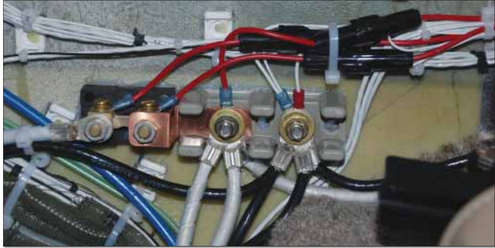
High-current wiring is part of the Therm-X installation; proper techniques are critical to the performance of the system.
